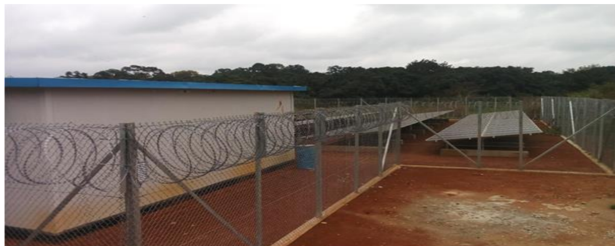
Site 3: solar mini-grid plant that can power various levels of cassava processing to be linked to power cassava processing from nearby farmer cooperatives in the Yoko council site.
